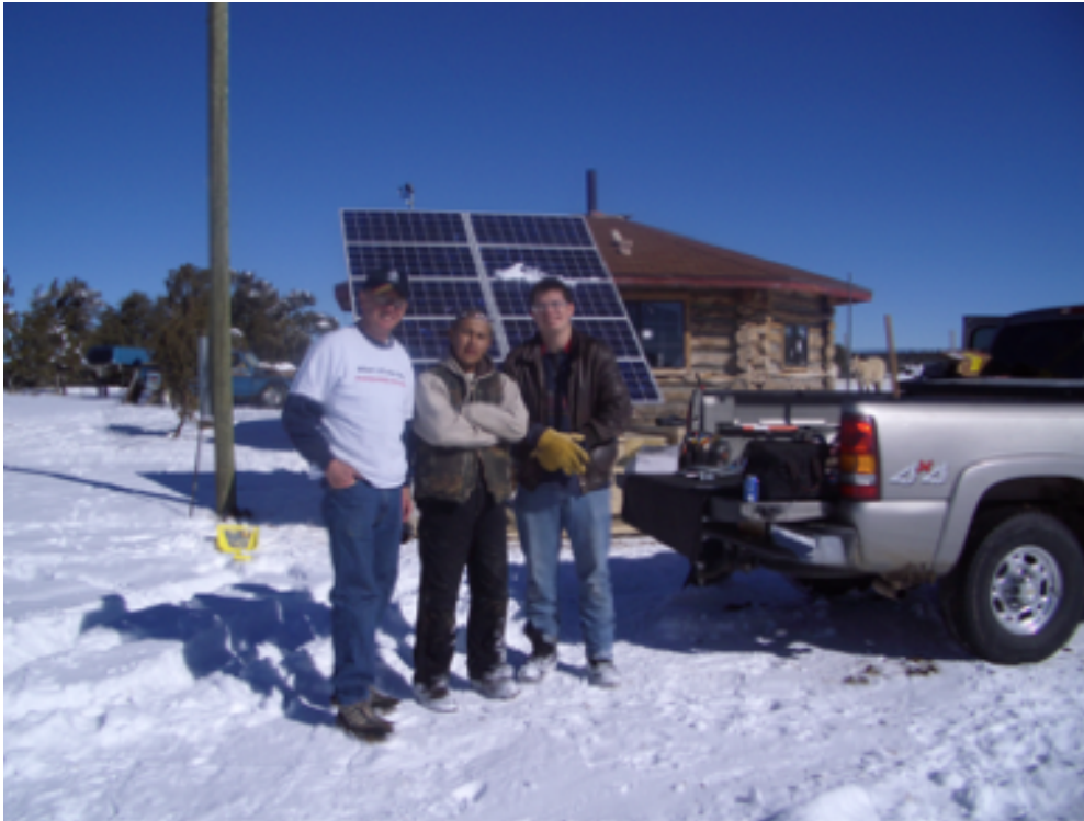
Figure 8. Installation of a small 800-Watt solar panel for a Hogan at the Ramah Navaho Reservation in western New Mexico. The project was done with the Engineers Without Borders club at the University of New Mexico.
