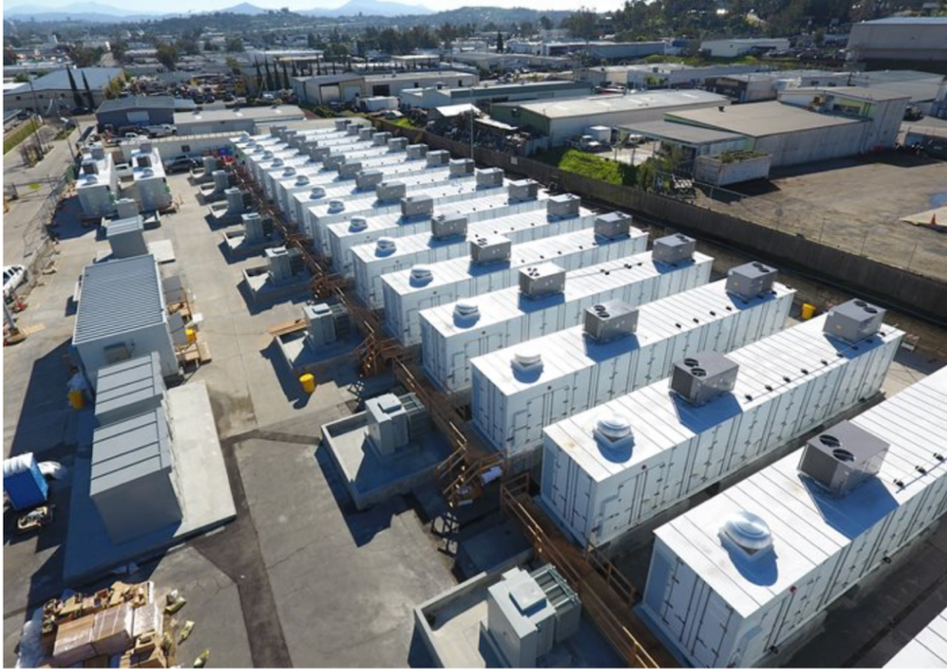
SDG&E's 30MW battery storage facility in Escondido, California. (Photo: San Diego Gas & Electric)
