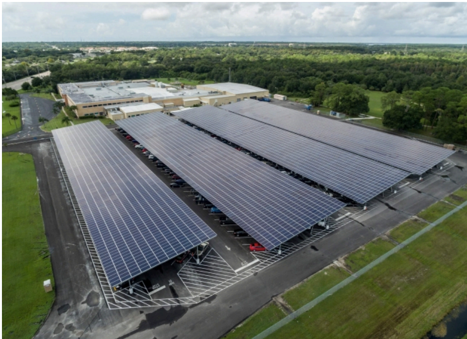
Figure 6. The parking lot solar system at the Lockheed-Martin Corp. facility in Oldsmar, Florida. The photovoltaic panels have a nameplate of 2.25 MW costing $5 million. The percentage of time that the system produces nameplate power per year is called the capacity factor and it is 17%.
